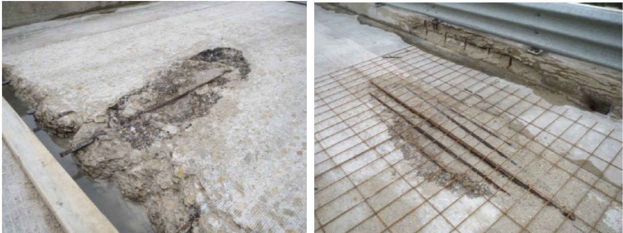
Figure 1. Examples of bridge deck distressed regions from Laporte Road bridge in Brandon, IA, before installation of UHPC overlay (adopted from: Haber et al. 2018)
